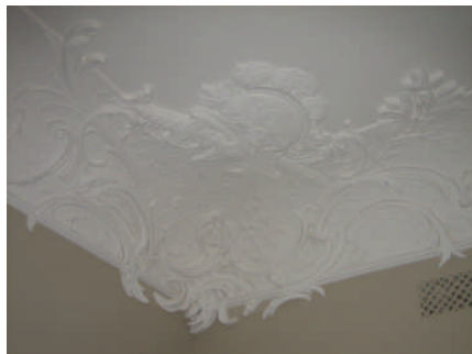
Cornice detail from RM Williams Heritage home, North Adelaide SA submitted by Coymans Ceilings
